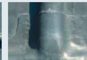
...closer inspection shows the capping soldered to the rolls, probably intended to prevent wind lift but only succeeding in restricting the natural thermal movement of the sheet, which will ultimately cause failure and water penetration.
