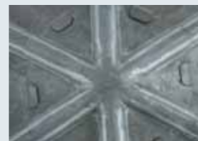
Properly formed crown capping, a complicated detail, neatly bossed and correctly clipped to prevent wind lift, with expansion gaps to allow natural thermal movement. Carried out by an LCA member, vetted and approved
