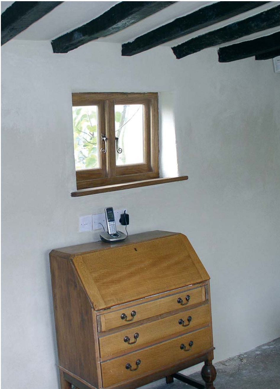
Above: Nearly finished. The casein paint has been applied and all that remains is to finish the rest of the room!
