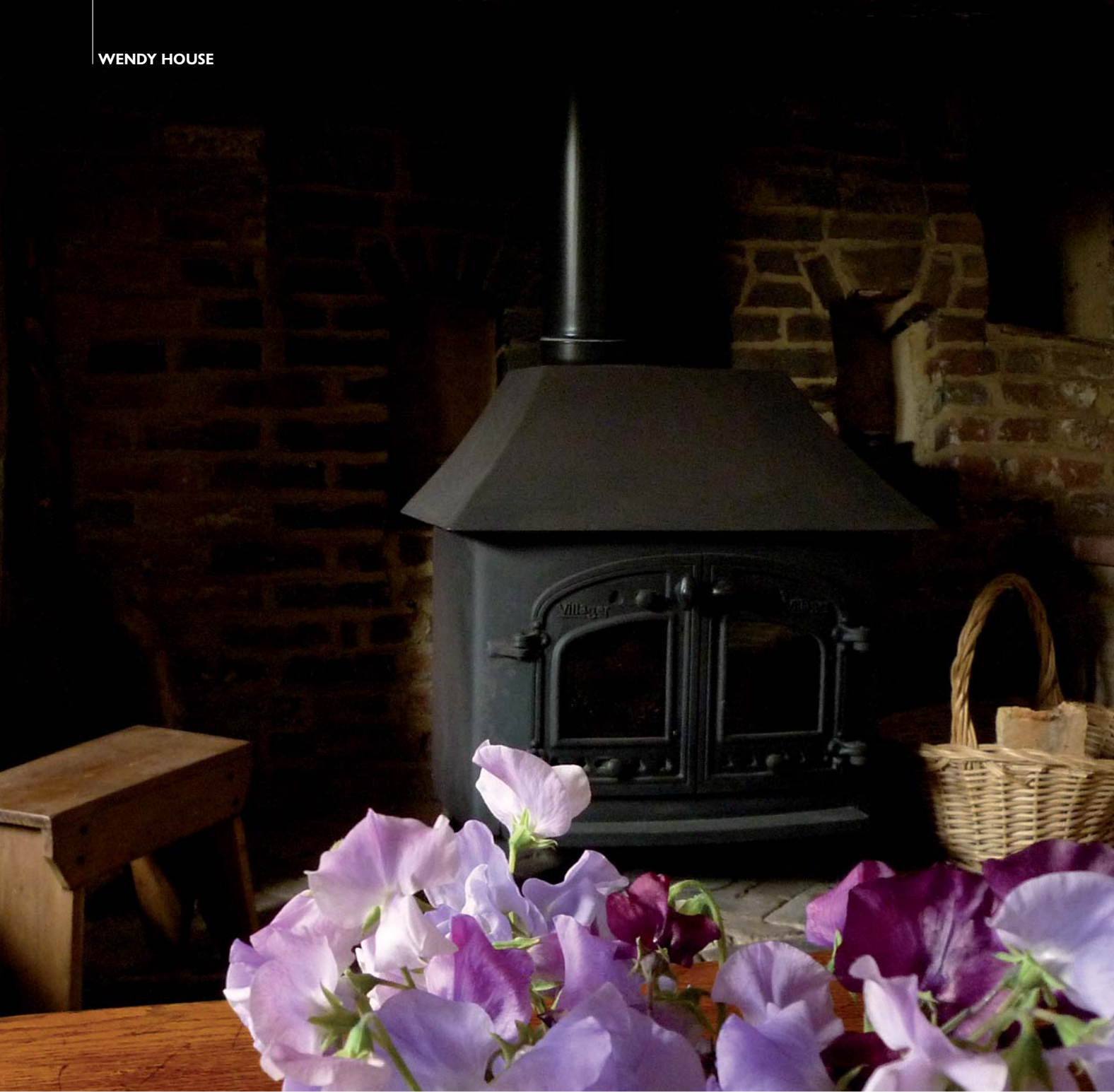
Wendy removed a complete modern fireplace to reveal the brick inglenook. She repointed, and in some instances replaced, bricks. One whole pillar had to be rebuilt, using back fill the she found at the rear of the fireplace
