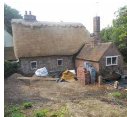
▲ The rear as it is now. Some 20 lorry loads of earth were removed at the rear of the cottage for the building – the site of the kitchen extension and the paved area and terraced garden beds.
